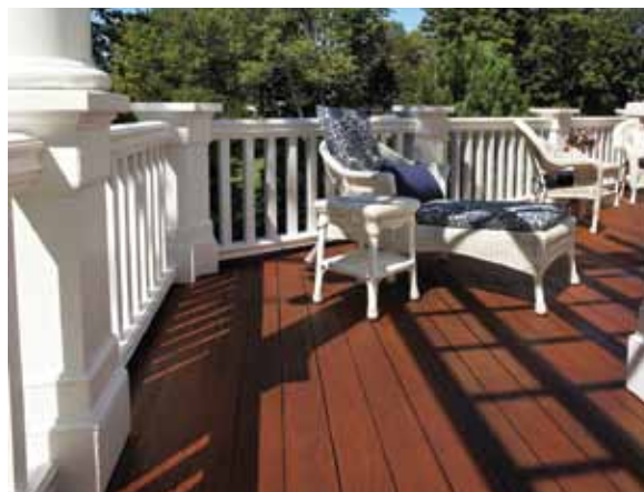
● This deck features Cabot® Australian Timber Oil in Jarrah Brown. The railings are in white solid color stain.
